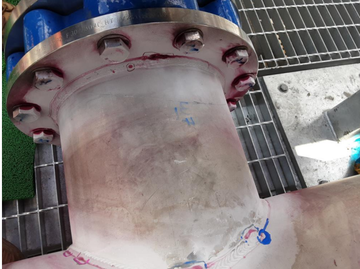
Image 9 of 13 - BTM SP3 W7: 4 off locations lack of fusion 6, 12, 3 o'clock up to 100mm facing west
