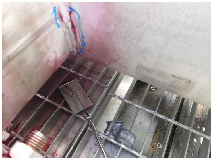
Image 8 of 13 - BTM SP3 W4: Intermittent Lack of fusion entire weld length up to 150mm
