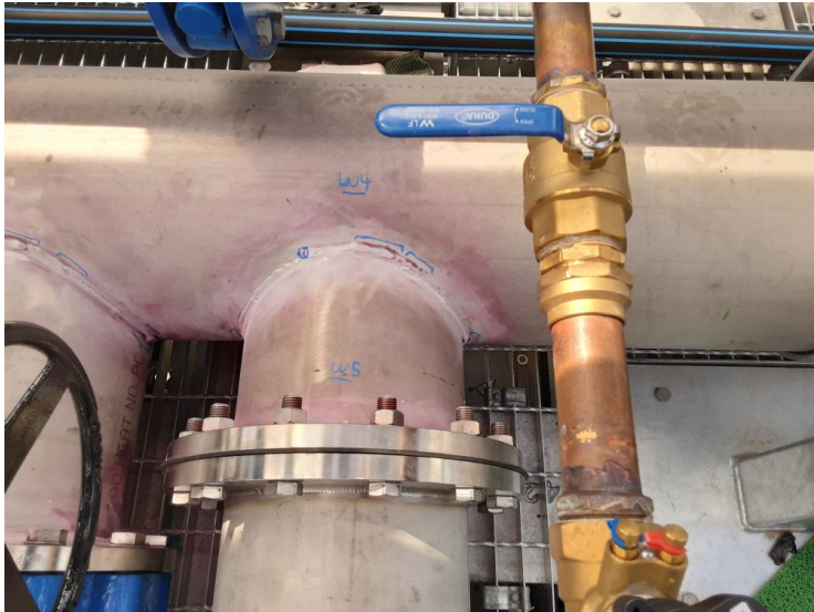
Image 5 of 13 - BTM SP3 W4: Intermittent Lack of fusion entire weld length up to 150mm
