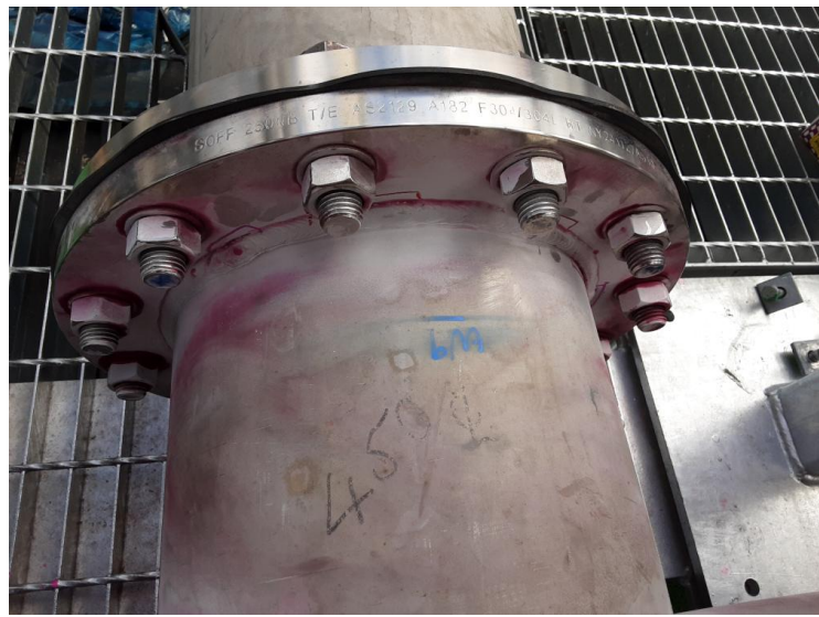
Image 12 of 13 - BTM SP3 W9: Intermittent Lack of fusion entire weld length up to 80mm
