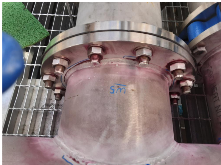
Image 4 of 13 - BTM SP3 W5: Intermittent Lack of fusion entire weld length up to 200mm
