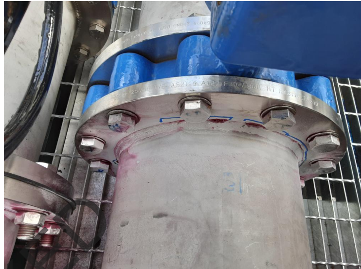
Image 6 of 13 - BTM SP3 W3: Intermittent Lack of fusion entire weld length up to 200mm
