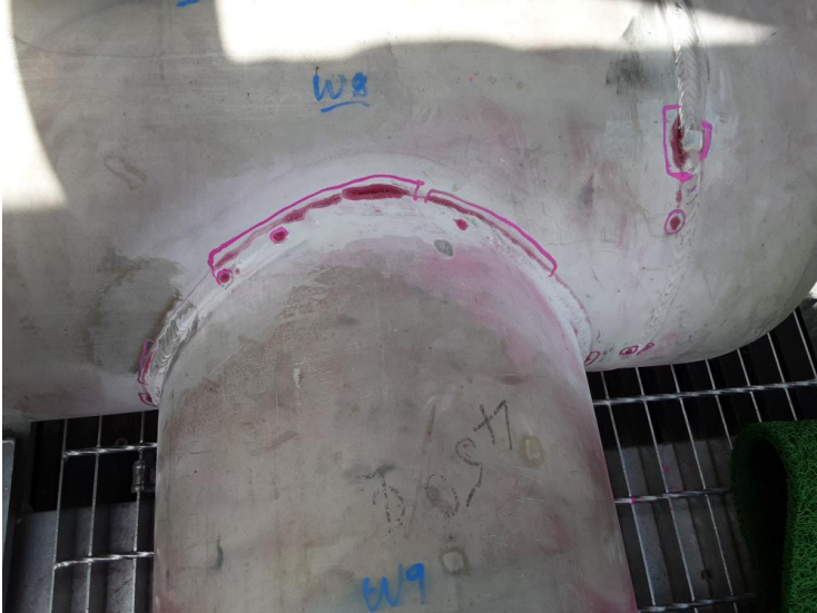
Image 13 of 13 - BTM SP3 W8: Intermittent Lack of fusion entire weld length up to 200mm
