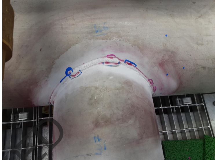
Image 10 of 13 - BTM SP3 W6: Intermittent Lack of fusion entire weld length up to 100mm
