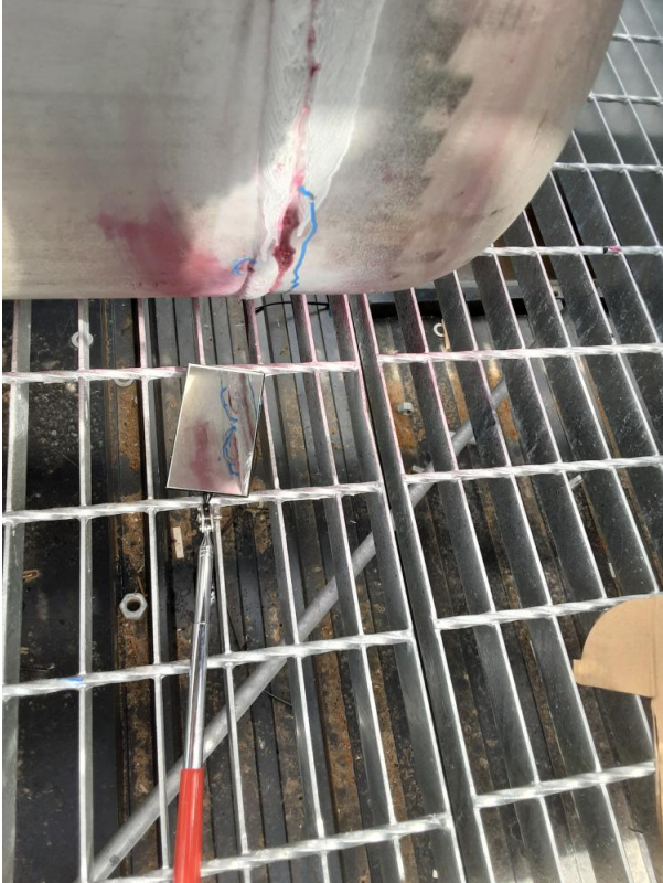
Image 1 of 13 - BTM SP3 W1: Lack of fusion areas 3-6 o'clock facing north
