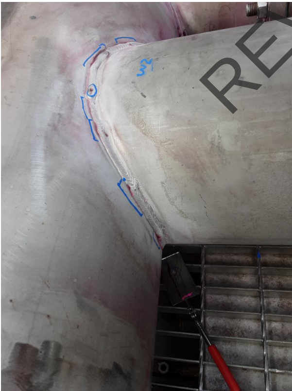
Image 7 of 13 - BTM SP3 W2: Intermittent Lack of fusion entire weld length up to 200mm
