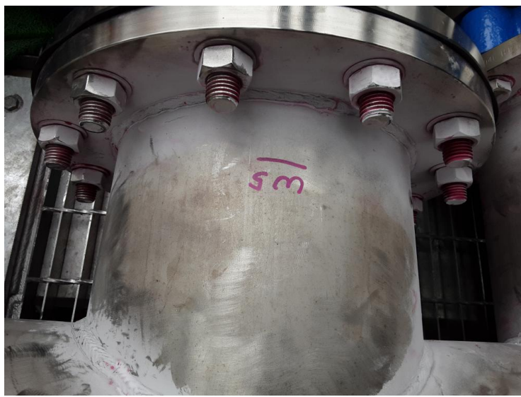
Image 4 of 11 - W4: 7 off indications @ 1, 3, 5, 7, 8 and 9 o'clock facing east
