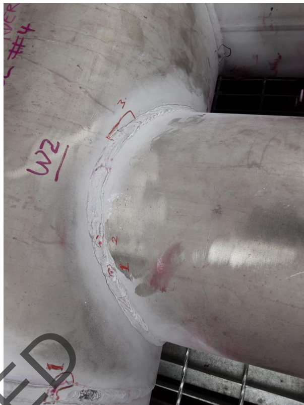
Image 2 of 11 - W2: 4 off indications @ 11, 1 and 6 o'clock facing east
