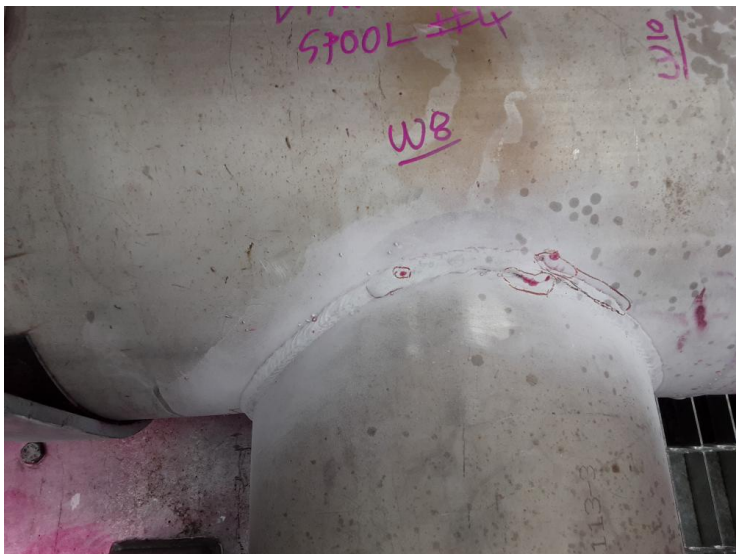
Image 11 of 11 - W8: 6 off indications @ 9, 11, 1, 3 and 6 o'clock facing east
