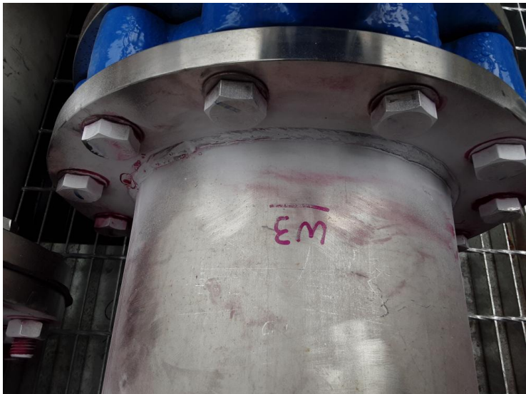
Image 1 of 11 - W3: 5 off indications @ 8, 9, 5, 7 and 3 o'clock facing west
