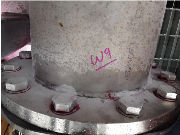
Image 9 of 11 - W9: 3 off indications @ 4, 11, and 7 o'clock facing west
