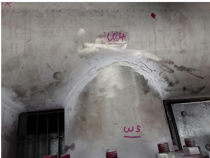
Image 5 of 11 - W5: 5 off indications @ 9, 3, and 5 o'clock facing west
