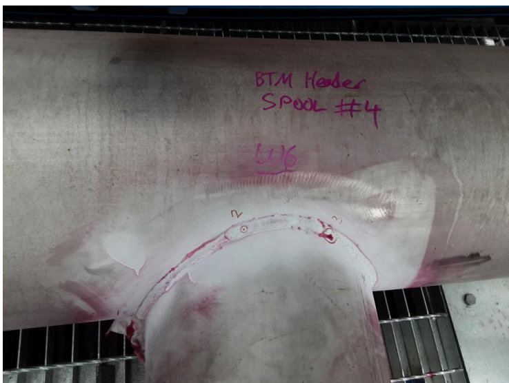
Image 7 of 11 - W6: 3 off indications @ 9, 11, and 12 o'clock facing east
