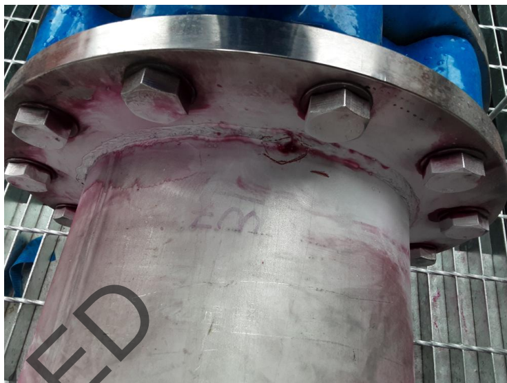
Image 6 of 11 - W7: 5 off indications @ 12, 9, and 6 o'clock facing west
